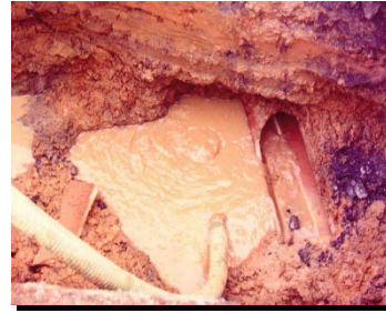
Hidden leak running into drain tile
