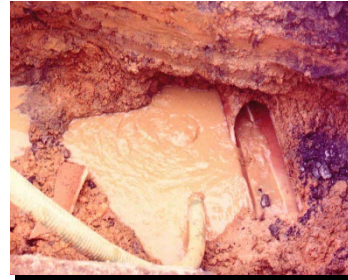
Hidden leak running into drain tile
